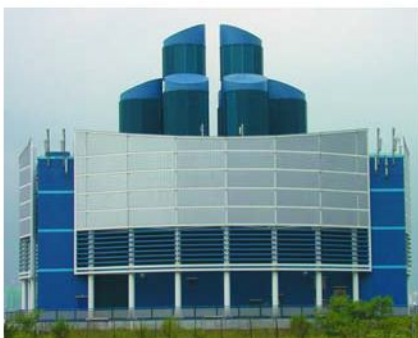
Western Harbour Tunnel, Hong Kong. Triple bank faceted circular louvre installed to handle the high air volumes required and to provide maximum rain protection even in typhoon conditions.
